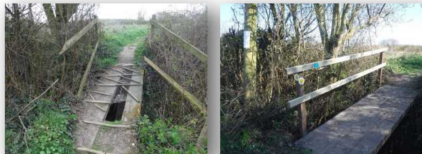
Bridge replacement by the Ramblers at East Carlton assisted with ongoing development of Kett's Country long distance Trail
