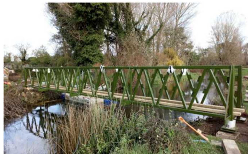
Completion of works on Angles Way bridge repair allowing route to be put back onto its original line
