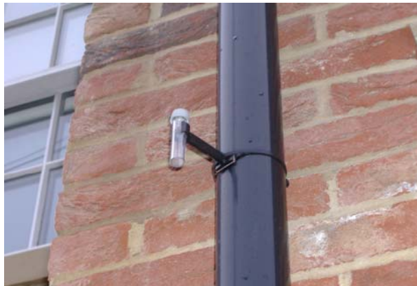
Tube mounted on rain water down pipe
